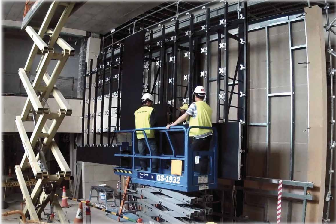
A work in progress: Techtel mounts the LED screen tiles to the frame one by one
